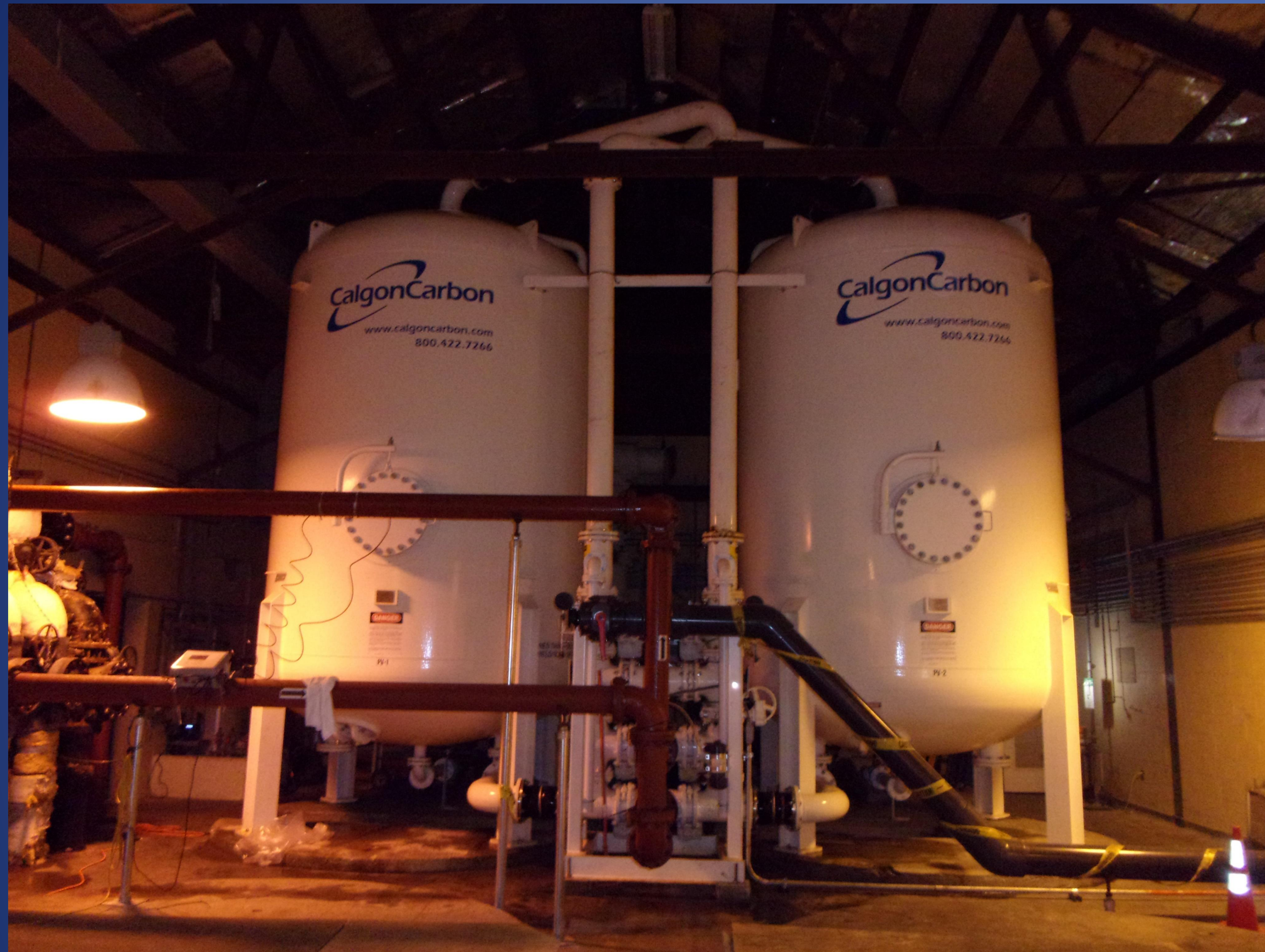
Pease Demonstration WTP GAC Units
