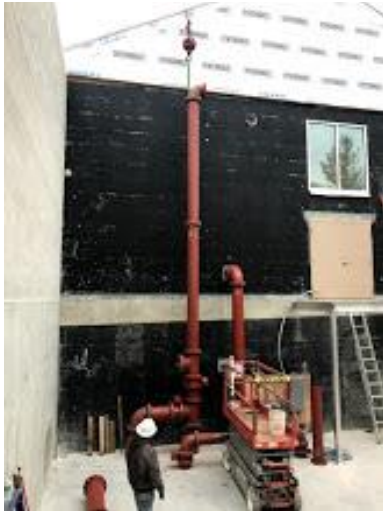
Figure 7-Inside Well 7/8 PFAS WTP Addition
