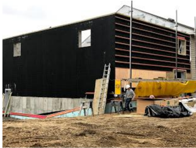
Figure 8-Exterior of Well 7/8 PFAS WTP Addition
