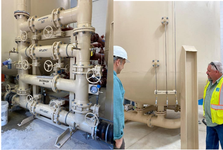
Figure 5-GAC Vessel Pipe Rack & Sample Taps-Well 4/5 WTP
